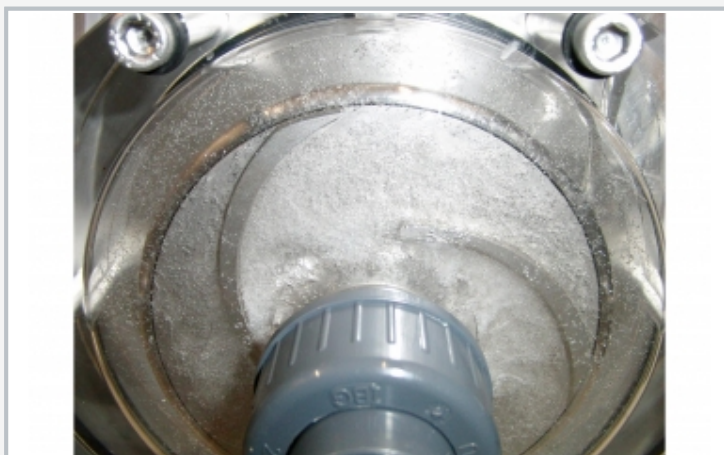
Formation of vapour bubbles due to cavitation at the pump impeller
